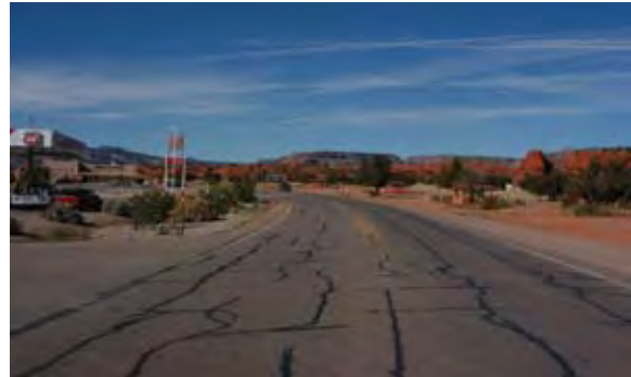
Looking north along NM 4 at the Red Rocks recreational area. Roadside land uses include the commercial area (service station and Walatowa Visitors Center) visible at left, and the recreational area (where small-scale vending takes place during the summer) at right. The speed limit along this segment of the highway is 50 mph.
